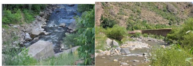
Figure 6. Yeghegis River banks sections that need strengthening.
