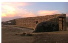
Picture 1. Passive solar greenhouse under construction in Kut, Gegharkunik region, Armenia. © RBHS
